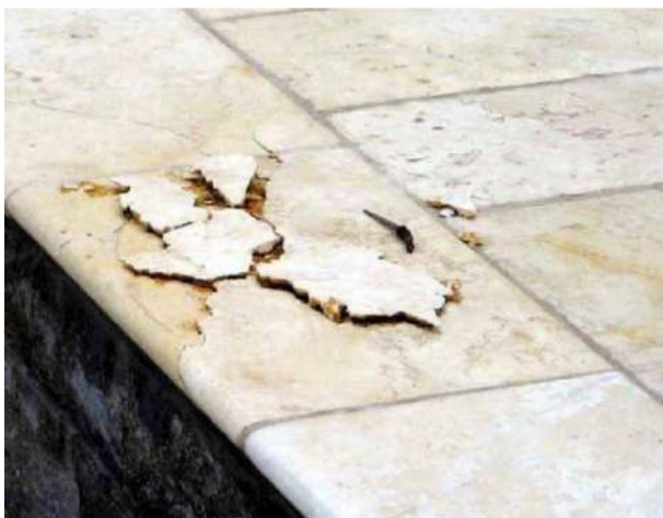
Figure 1: Damages due to saturated freeze – thaw cycling of a limestone paving [58].
