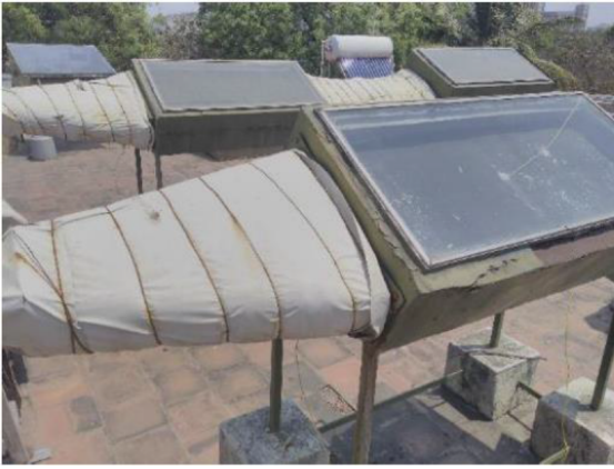
Figure 3: Inlet connected to the blower.
