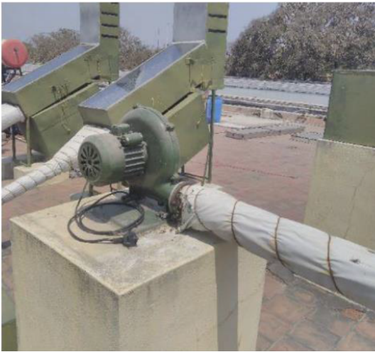
Figure 4: Blower connected to the inlet.
