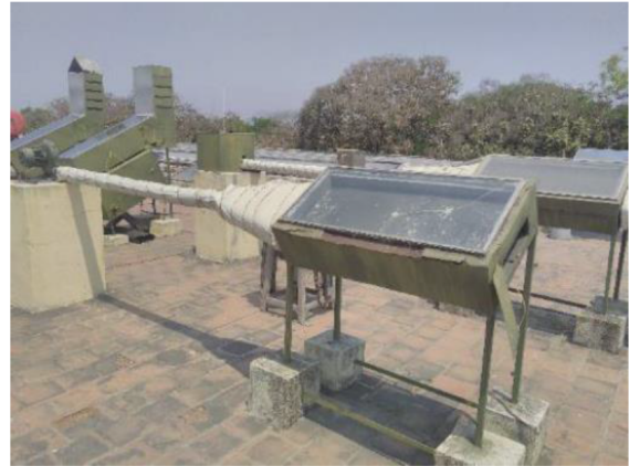
Figure 1: Solar air heater with a glass plate and absorber plate with an inlet connected to blower and outlet on the other end.
