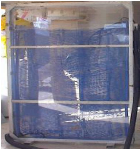
Figure 3: Photo of the air-conditioning cupboard.
