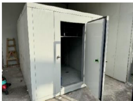
(a) Exterior of the cold store
