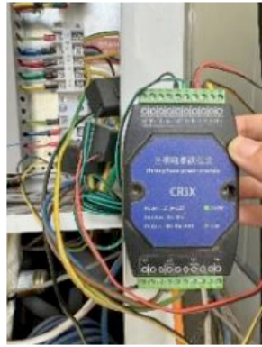
(a) Electricity metering modules
